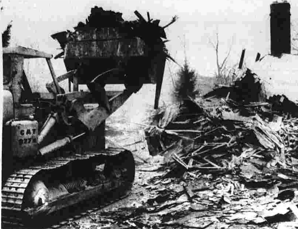
A bulldozer from Fava's Building Wrecking Co. of Middletown demolishes an abandoned house at 14 Shallowbrook Lane. It was the site of many set fires and considered a hazard to the community. (Herald photo by Pinto)
